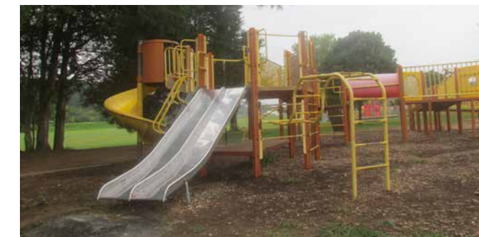
Grass and packed earth are unacceptable playground surfaces.
