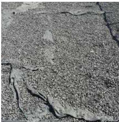
Geotextile fabric should never be exposed and is a sure sign that surfacing levels are inadequate.
